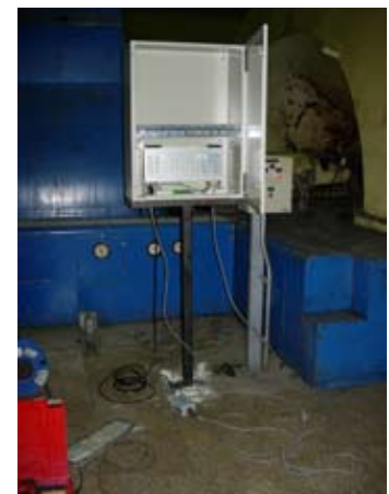
Image 3- Telemetry receiver installed into a box
